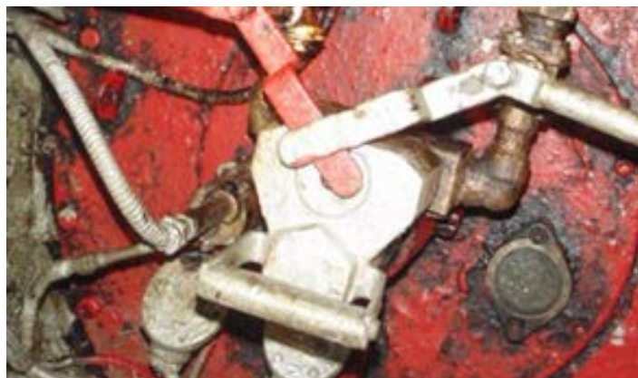
Figure 2: Missing screening of boiler fuel piping connections
