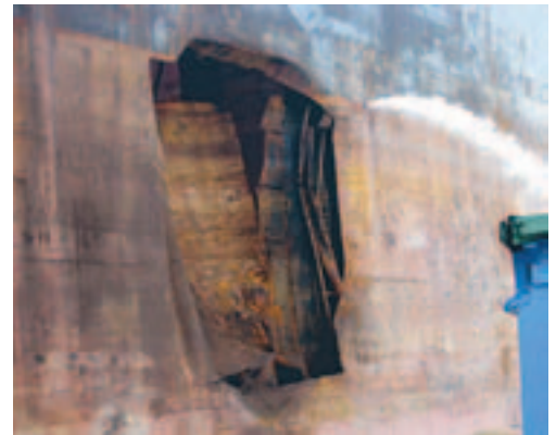
The damage, showing clearly how the bulb of the opposing vessel protruded through the hull.
